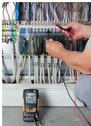
Testing voltage in a switching cabinet.
