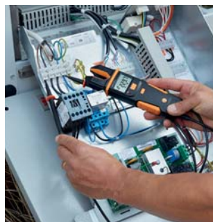
Measuring voltage on a compressor.
