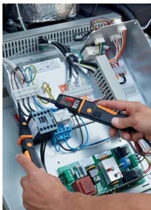
Measuring voltage on a compressor.
