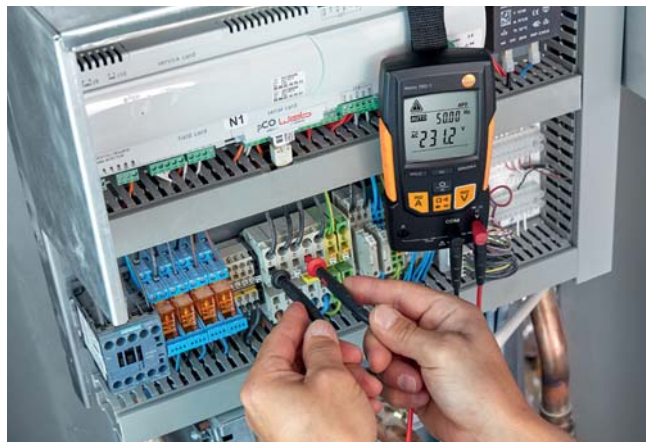
Testing voltage in the switching box of a heat pump.
