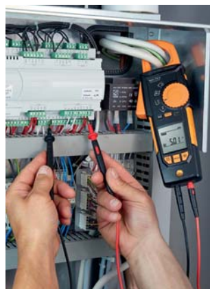
Measuring voltage on the switching box of a heat pump with suspended measuring instrument.
