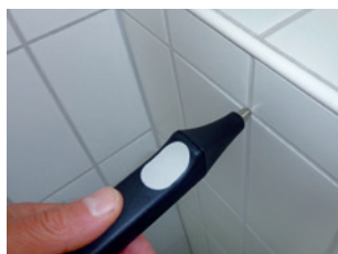
Localization of water damage through narrow bores.
