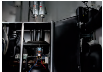
Analyze heat pumps
