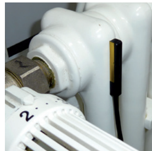
Measurement on a radiator
